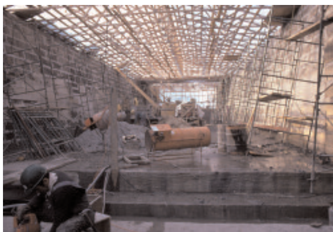
Five of the eight locks in flight at the Ottawa lockstation were reconstructed in the 1980s, 1986, Rideau Canal Archive.
