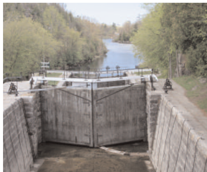
Lower lock gates at Kingston Mills and excavated channel to Lake Ontario, 2005, Simon Lunn.
